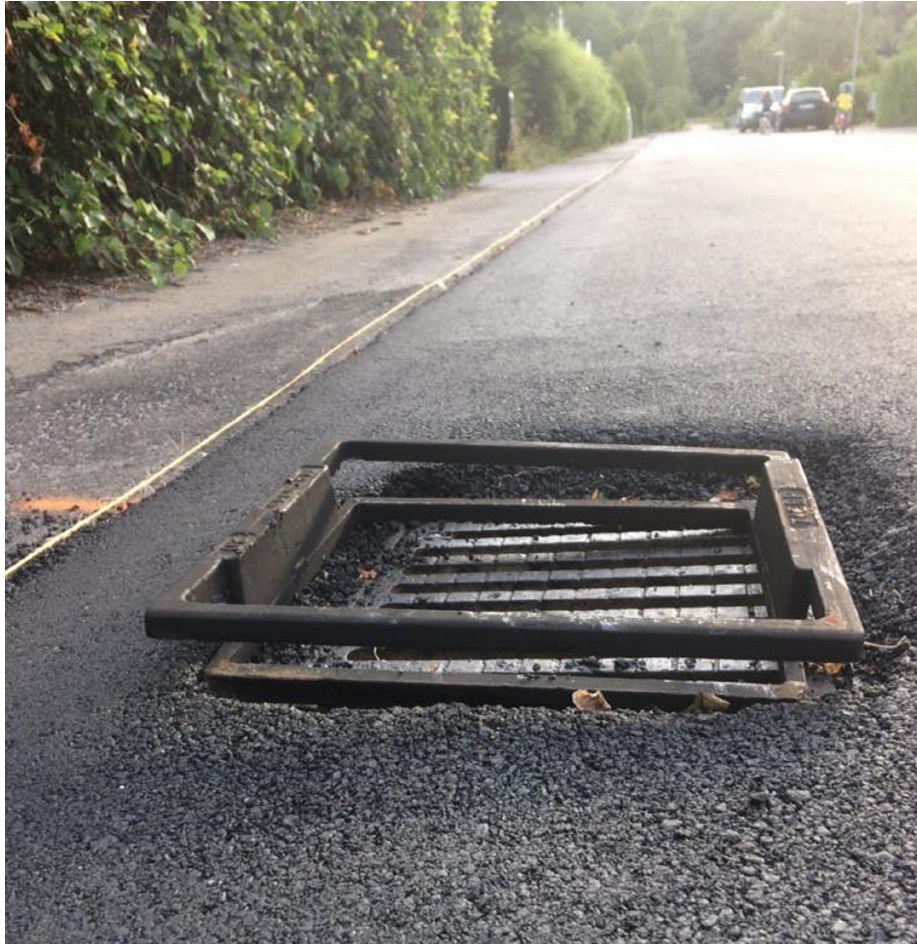
Figure 9 : Dangerous manhole cover in Sweden
