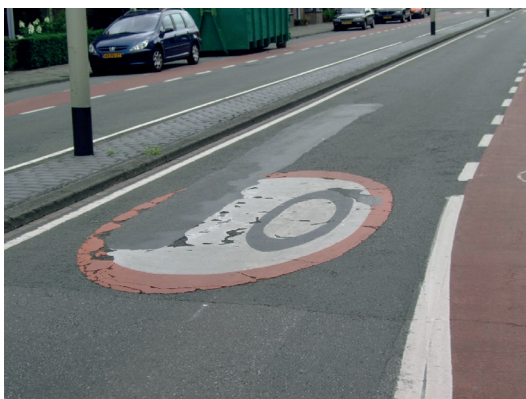
Figure 4: Badly maintained road marking
